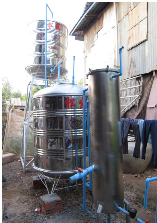
Figure 2. SARSAC system installed at Prek Chrey Khnong village of Kandal province, Cambodia.
